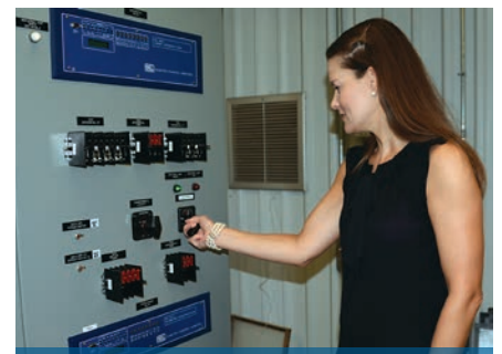
SLEMCO CFO Katherine Domingue turns the switch to energize our new U. J. Gajan substation.
