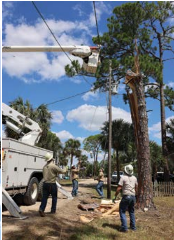
Hurricane Idalia brought significant damage and flooding across its path through the Southeast. Photos by Ralph Demillo
